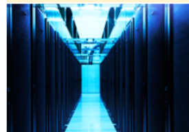
AI Bridging Cloud Infrastructure (ABCI) - PRIMERGY CX2570 M4, Xeon Gold 6148 20C 2.4GHz, NVIDIA Tesla V100 SXM2, Infiniband EDR
